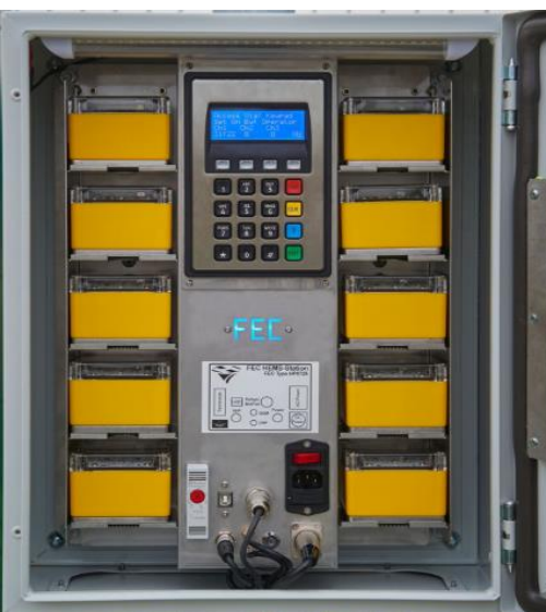
The Glenforsa Community Night Operational Temporary Landing Site, illuminated by the FEC HEMS-Station® system, provides a 24/7/365 critical care service on the Isle of Mull
